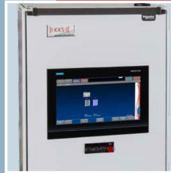
Touch Screen panel with overview of process tanks
